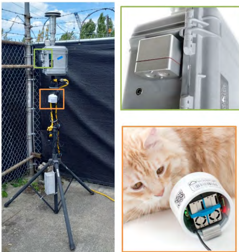
Figure G-1: illustration of the N-FRM installation at our UEWA (Fontanelle St.) site, with Purple Air sensor added to the setup(left). The other two photos (borrowed from Purple Air© and ARA instruments© websites), provide a more detailed look at the N-FRM RTP (upper right) and Purple Air sensor (lower right).
